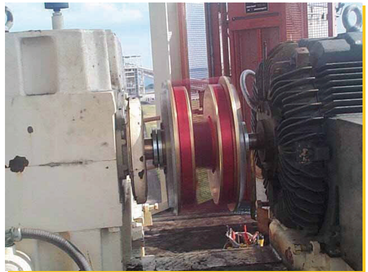
▲ MGTL 12/20, Power Generation, Conveyor System, TX, USA
