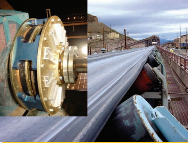
▲ MGD 20/400, 300HP, 1800RPM, Mining, Gear Box in Bulk Conveyor System, AZ, USA
