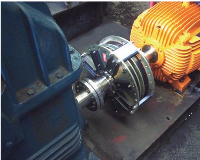
▲ MGD 18/250, 150HP, 1500RPM, Steel Mill, Conveyor System, Australia
